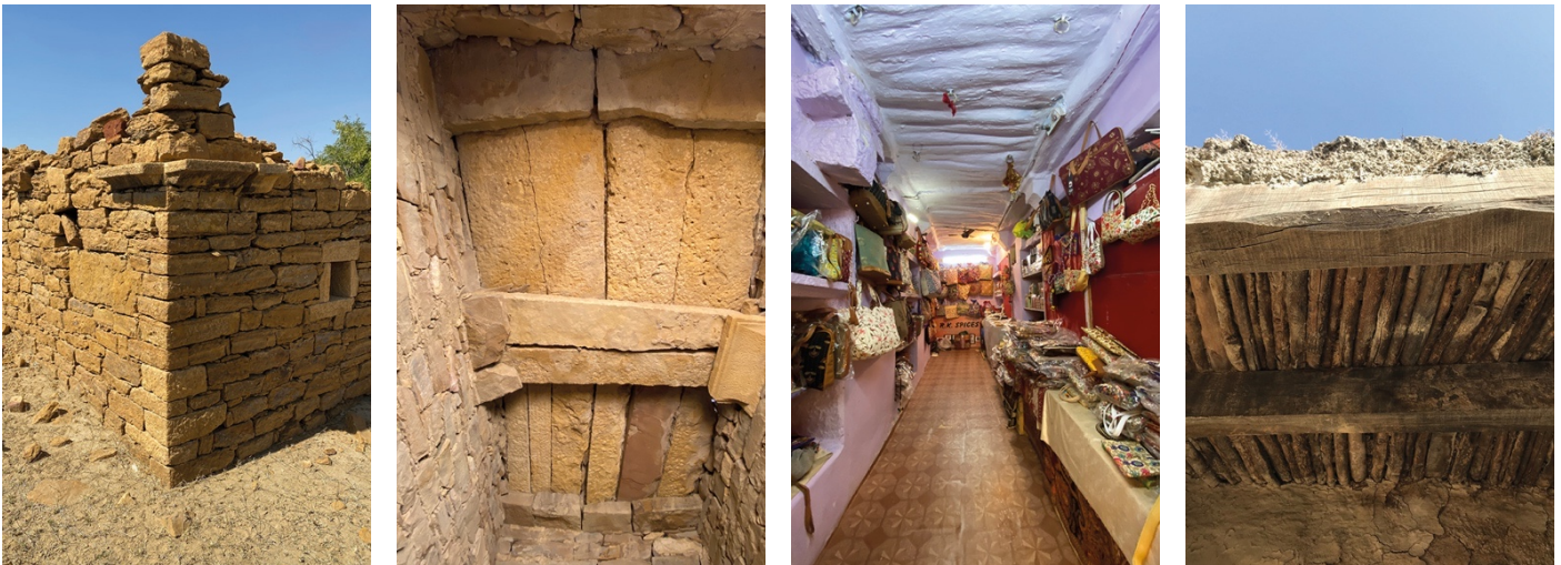
Figure 15 Use of stone brackets with stone pattis and wooden beams to span spaces
