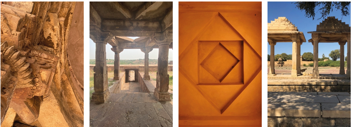
Figure 16 Rudimentary form of corbeling seen in the roofs of religious and public buildings in the region.
