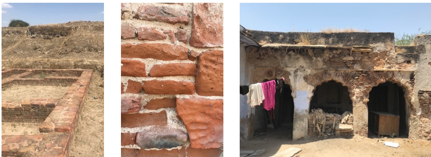
Figure 10 Various form, size and types of mud bricks used for walls and arches around Jaipur district, Rajasthan
